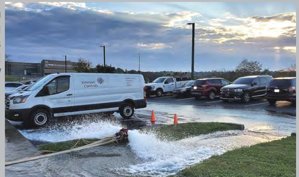
A beautiful day for a fire pump test at Kentucky State University!
